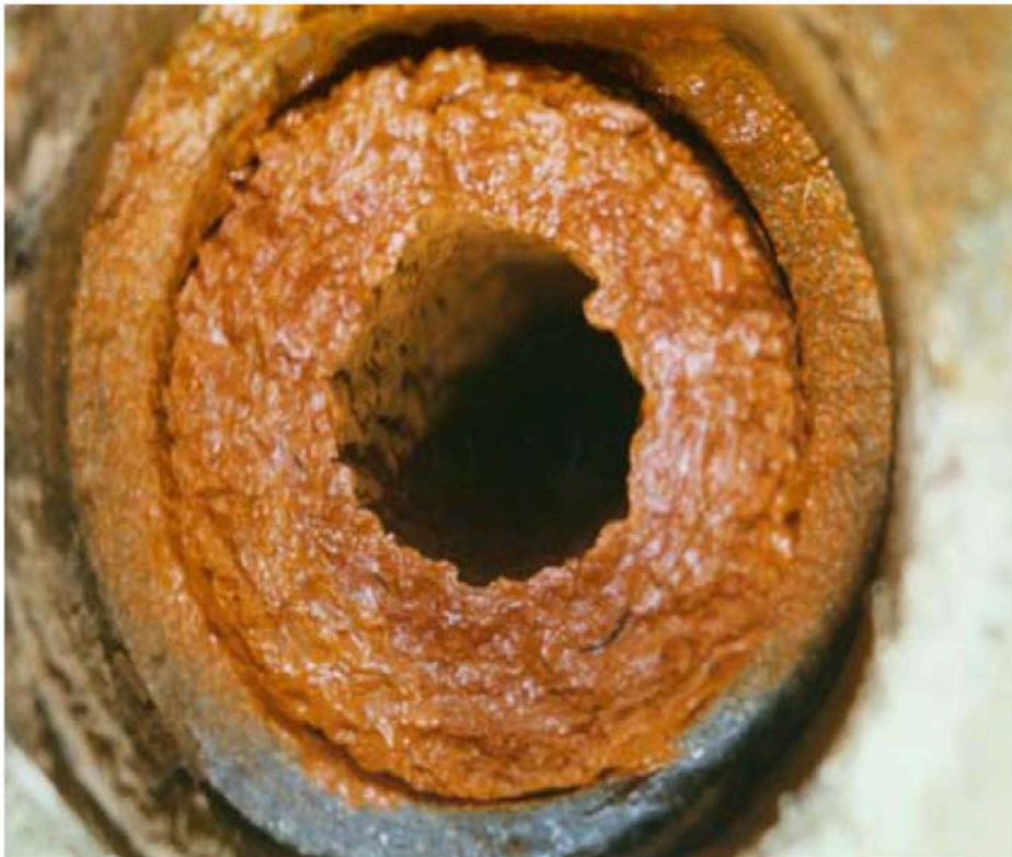
100 mm pipe clogged with an iron bacteria biofilm. Source: SA MDB NRM Board (2006).
