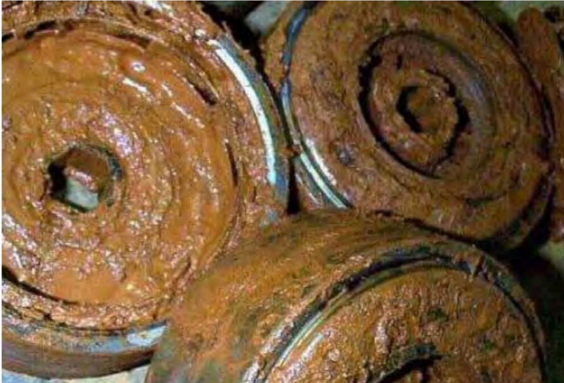
Iron biofouling of a submersible pump. Source: Forward (2008) in GHD (2010).
