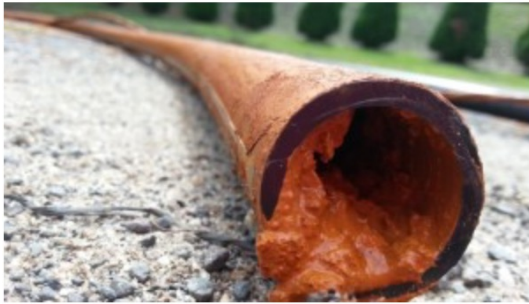
A dripper line from the Limestone Coast region affected by iron sludge.
