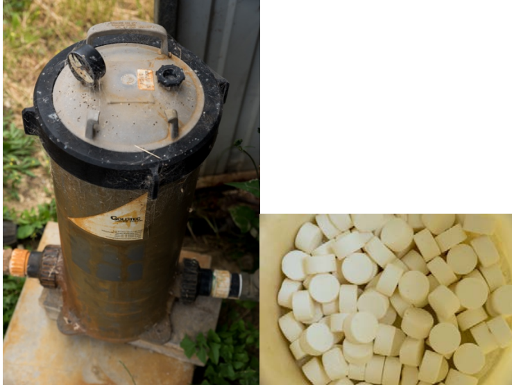
A chlorination system used in the Limestone Coast region, showing the automatic dosing unit and chlorination pellets. Photo: Gavin Blacker.
