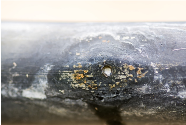
Calcium carbonate scale build-up in a drip line.
